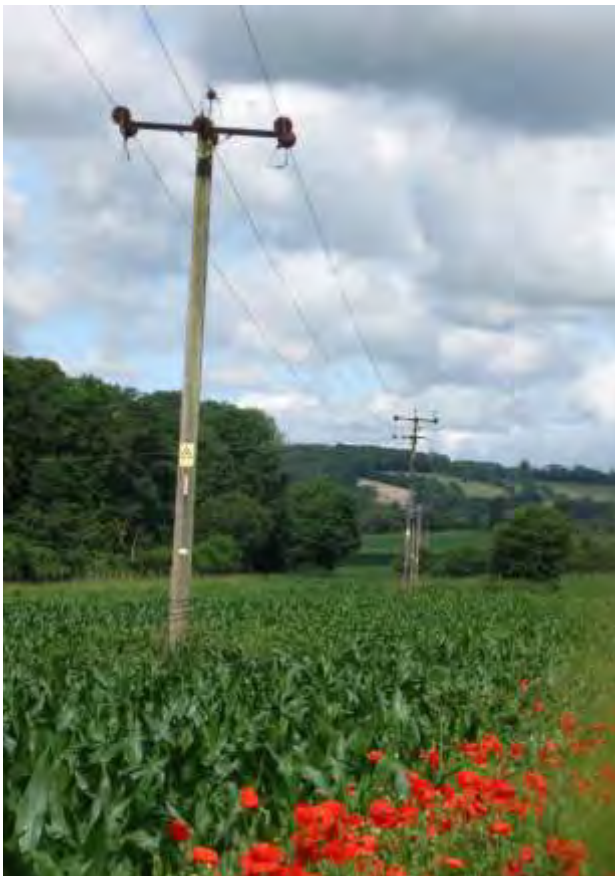
Turville - overhead wires that are a good candidate for removal
