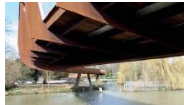
No maintenance Corten structure on 180m long footbridge; University of Northampton, Waterside campus
