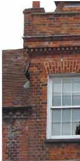
Rubbed, cut and moulded bricks used to corbel out base of parapet (Wendover)
