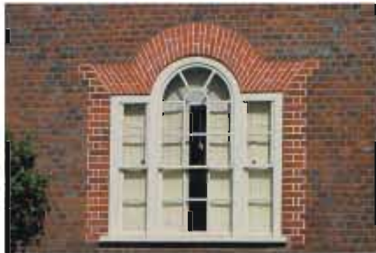
Contrasting mortars used to great effect to distinguish dressings (using lime putty on the arch and tuck pointing to the quoins) from the main elevation brickwork in black mortar
