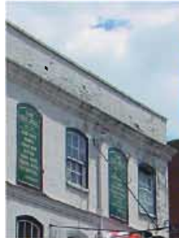
Painting brickwork creates its own maintenance problems
