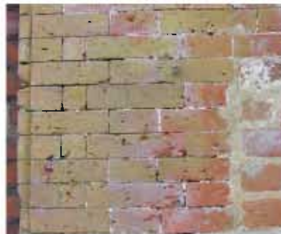
Finely gauged brickwork (Hemel Hempstead). Note the difference in joint width in the repaired area.
