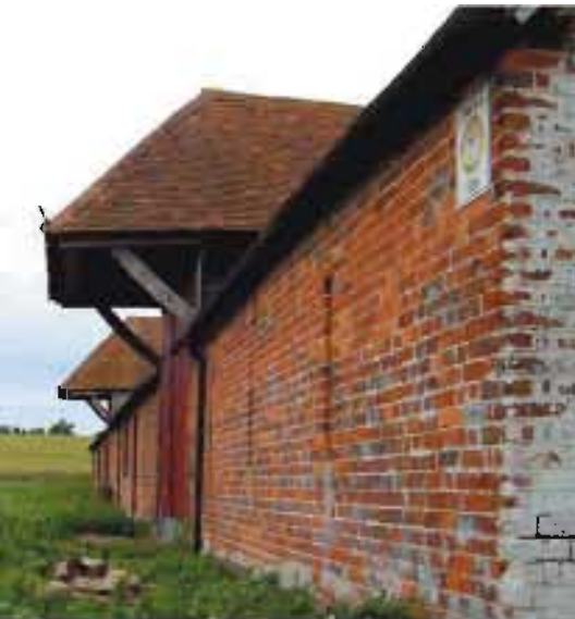
Brick was used for the walls of this massive threshing barn (Ipsden)
