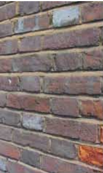
Weathered pointing overemphasises the horizontal joints by creating shadow lines
