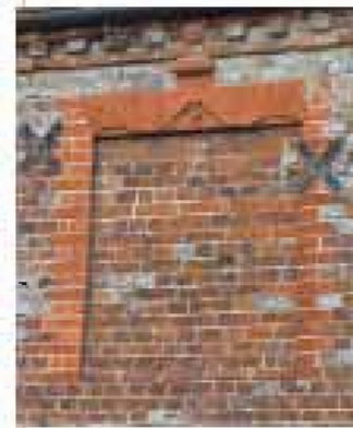
Blocked window with elegant scrolled lintel. Note also the dentil cornice detail (Wendover)
