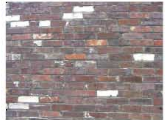
The poor use of reclaimed bricks detracts from the appearance of this brick elevation
