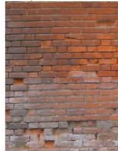
Differential weathering of bricks (Piccotts End)
