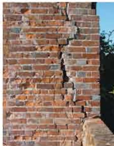
Brickwork in poor repair
