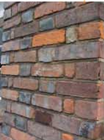
Double struck or beak pointing exaggerates the joints
