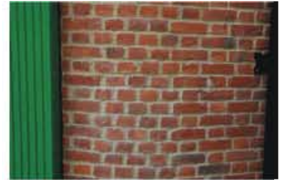
Modern brickwork marred by poor pointing (Wallingford) (Photo C. White)
