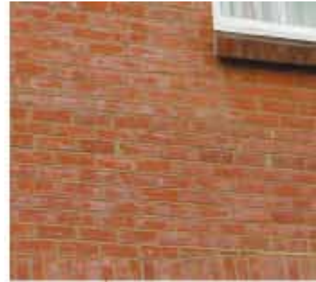
The effects of efflorescence
