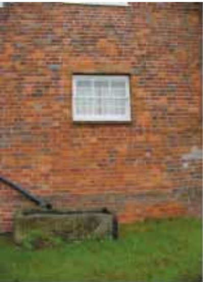
Patchwork repairs to brickwork using cement-based mortars are very difficult to disguise or reverse
