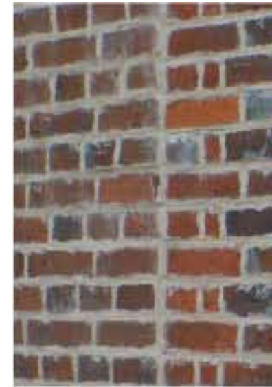
Messily applied lime mortar with a poor attempt at scored jointing
