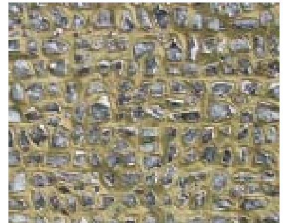
Poor mortar finish
