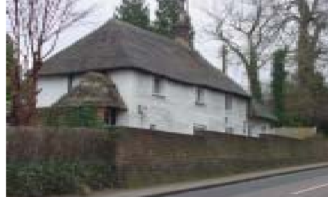
The painted flintwork and thatched roof is unusual in the Chilterns (Ellesborough)
