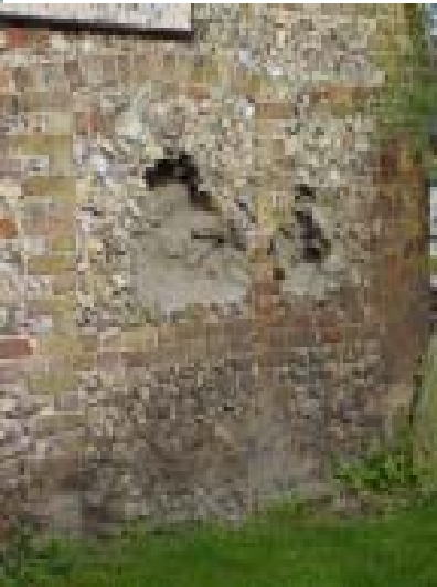
Flint in poor repair
