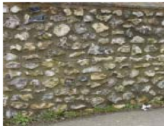
Cracking in hard cement mortar
