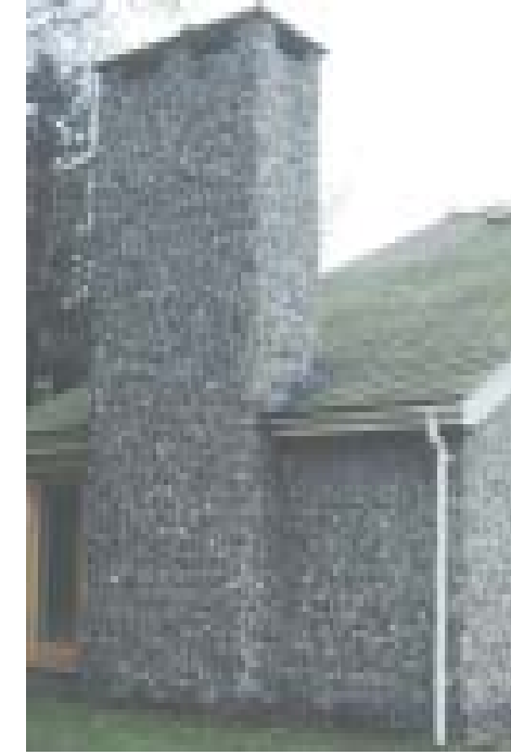
Impressive use of flint marred by poorly executed mortaring
