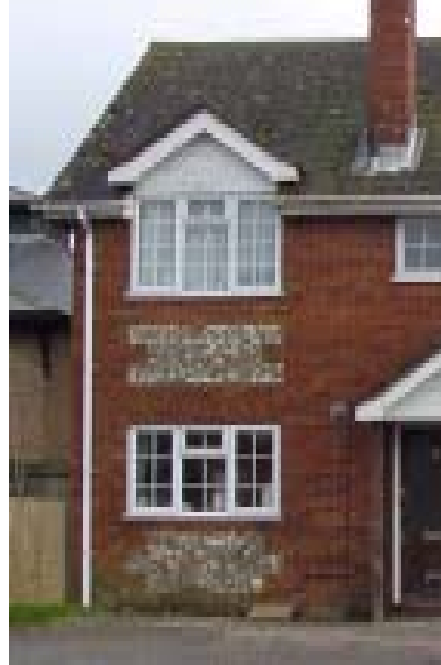
The token panels of flint do nothing to enhance the appearance of this poorly designed building
