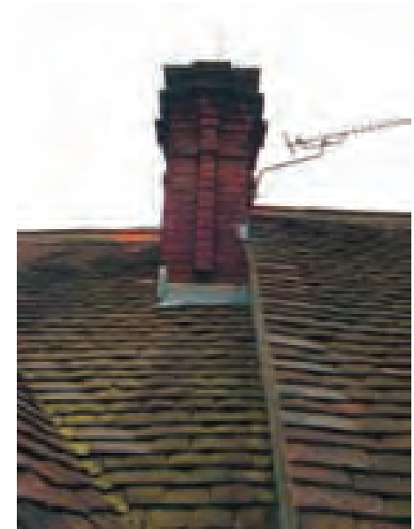
Contrasting verges – half-tile slips to left, tile-and-a-half to right. Note also the valley tiles (Tring)
