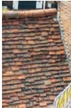
Tiled roof in poor repair (Hemel Hempstead)
