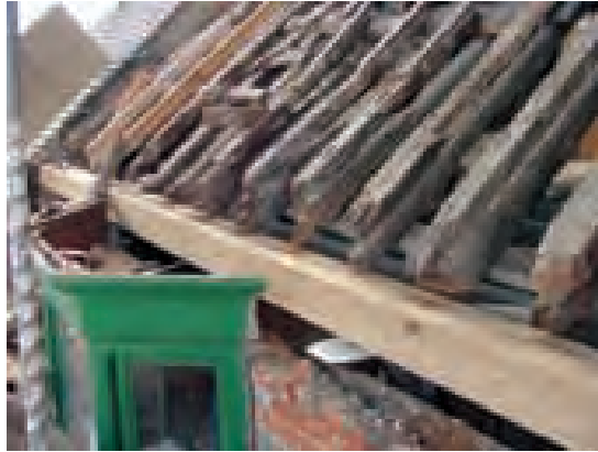
Roof timbers under repair (above) and roof being stripped (below) both at 173 High St., Berkhamsted
