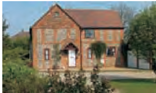
This roof demonstrates a failure to mix tile batches
