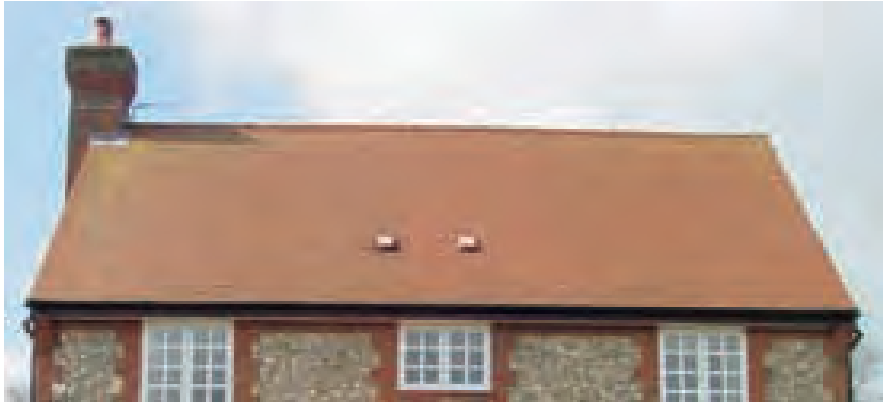
Ventilation tiles (near Stokenchurch)
