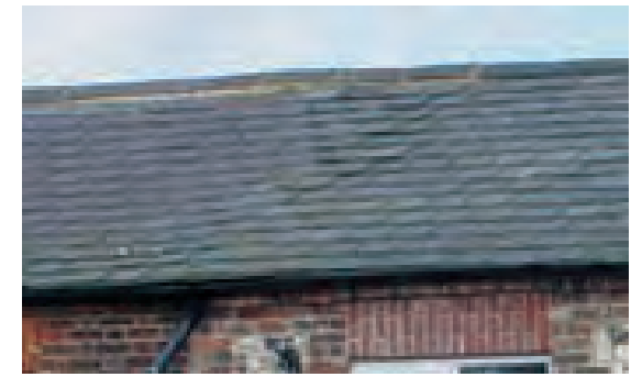
New slate roof to right poorly tied in to existing roof (Jockey End)
