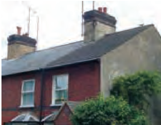
Changing roofing materials may impose additional loads on the roof structure and may detrimentally affect the character of the building (Hemel Hempstead)
