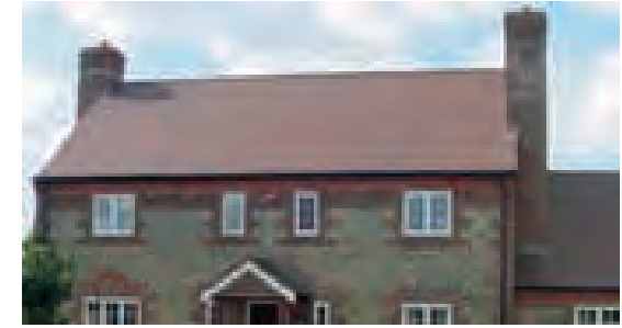
Machine-made tiles cannot match the subtle textures of hand made ones (South Chilterns)
