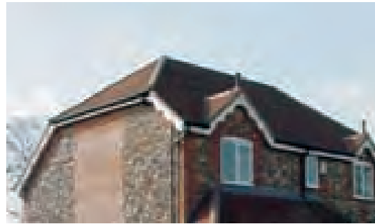
The incorporation of half hips in Chiltern roof designs can rarely be justified, particularly in conjunction with slender trussed roofs (Great Kingshill)
