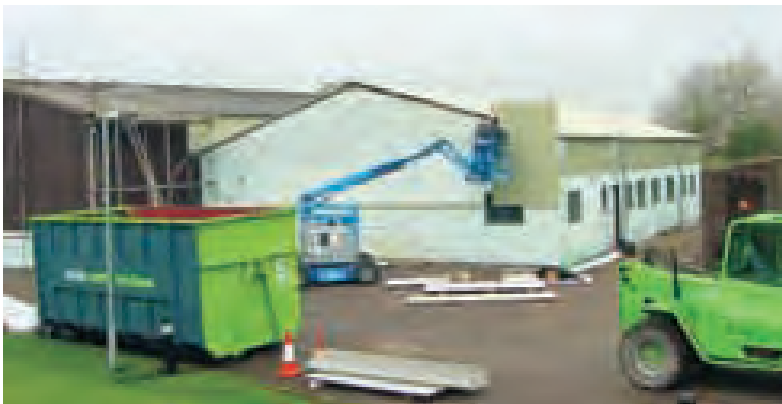
Roofing work requires rigorous health and safety measures to be in place
