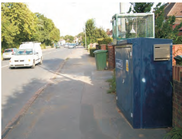
Temporary monitoring station installed as part of a programme to improve air quality in an AQMA
