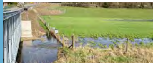
River water spilling into the floodplain through a damaged section of the bank of the R. Misbourne at Bottom House Farm Lane. Credit Allen Beechey
